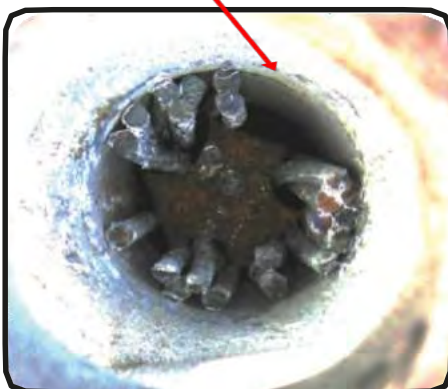
Incorrect Installation of Wedge
