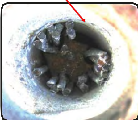
Incorrect Installation of Wedge
